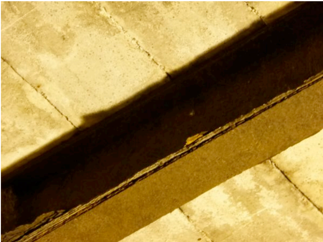
Corroding Roof Support Beam
