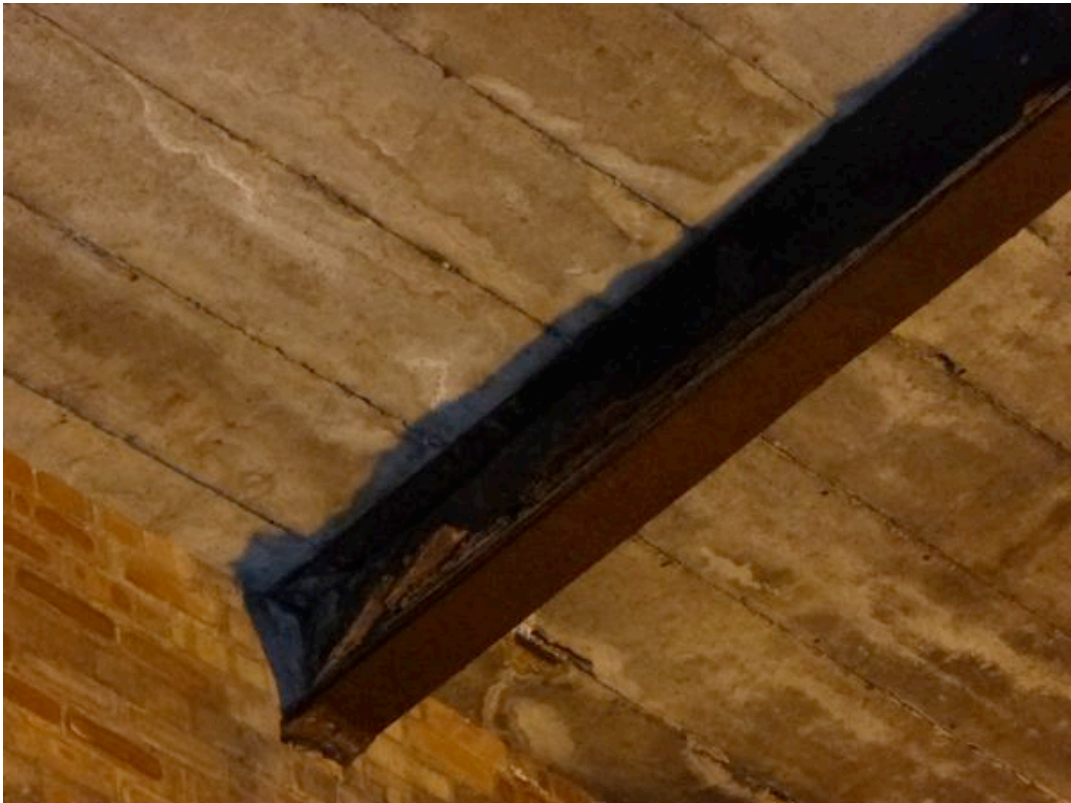
Corroding Roof Support Beam
